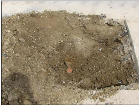
View of the top of the railroad rail as found.
