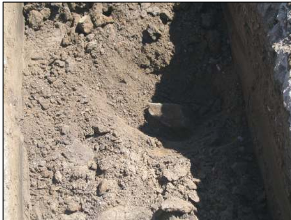
The stone found below the rail.
