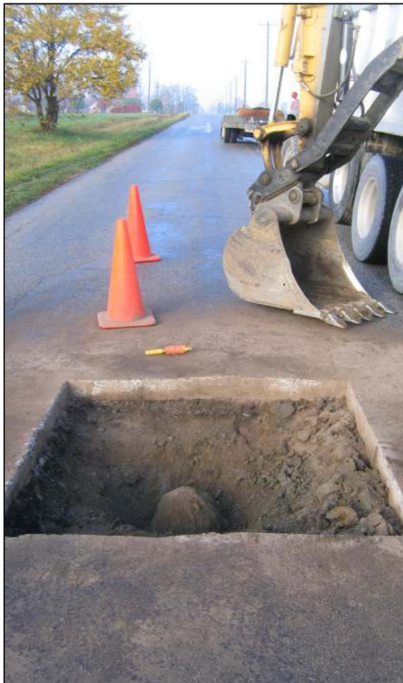
View from the east, looking across the stone and west along County Road 100 South.
