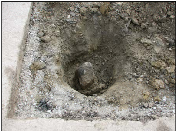
View of the stone after the rail was removed.
