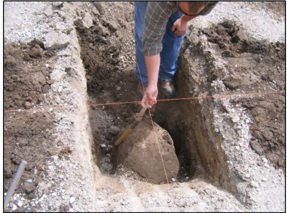
Brandon Miller holding the iron pipe in the approximate position as it was originally found and oriented, prior to removal.
