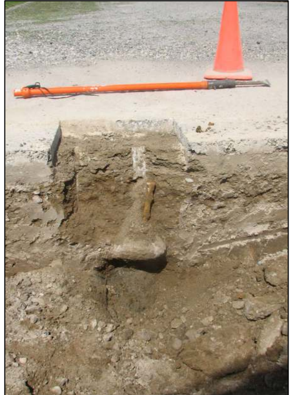
View showing the railroad spike (top), upper stone (middle), and lower stone (bottom)
