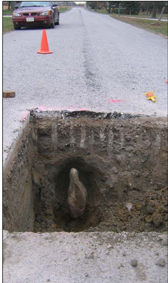
Corner stone. View from east of fully exposed stone and County Road 700 South to the west.
