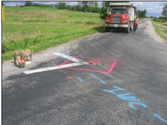
View from the west, looking across the stone and east along 166th Street in Hamilton County.
