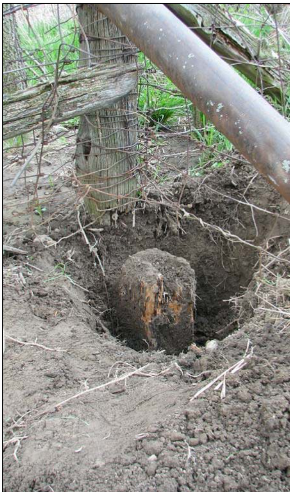
Base of old cedar post exposed. View from northwest.
