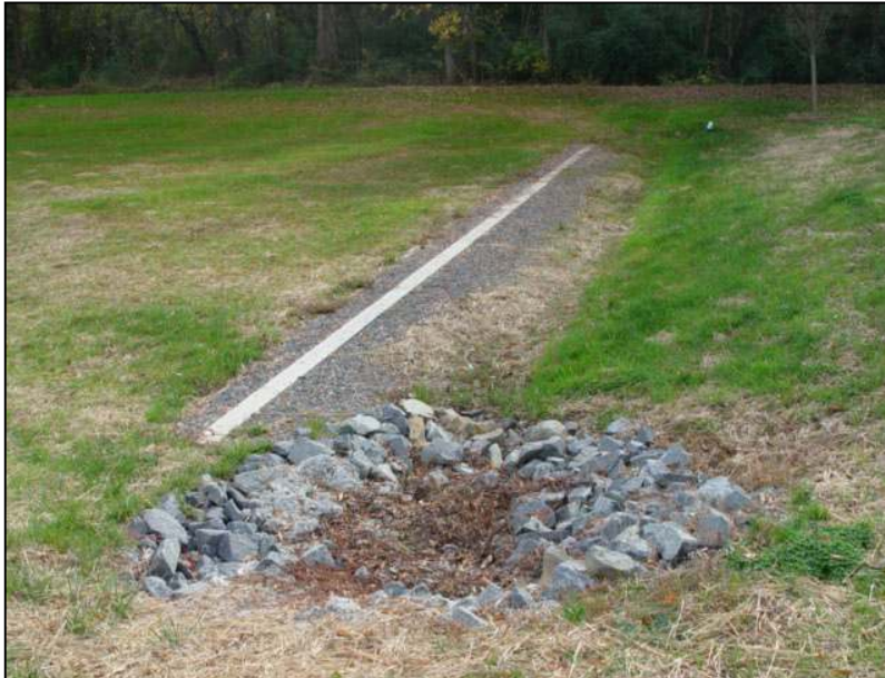
Figure 1 Level spreader, Charlotte, NC (NC State University)
