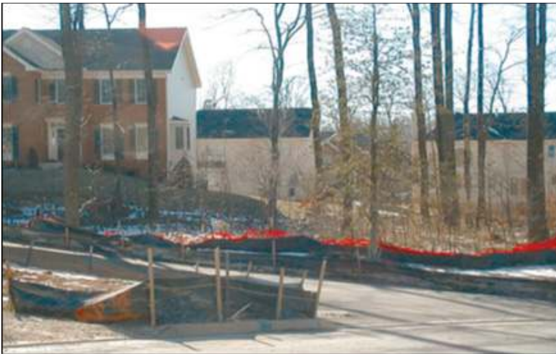
Figure 1 Undisturbed areas are protected during construction (Lake County, OH Stormwater Management Department)
