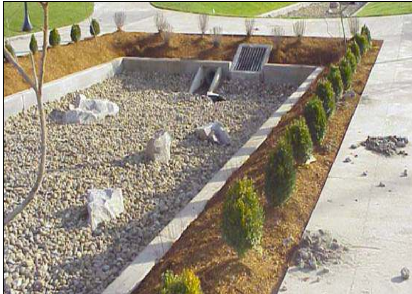
Figure 1 Constructed filter, Portland, OR (City of Portland 2004 Stormwater Management Manual)
